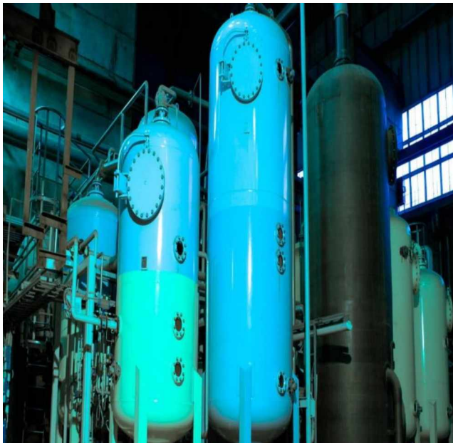
Filtered containment venting systems
