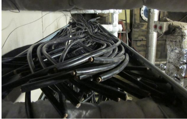
Fig. 2: Loose arrangement of the electric cables (CT2 test).
