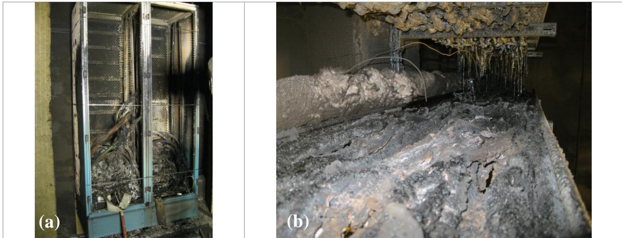
Fig. 23: After CFS-5 test. (a) Fire cabinet. (b) Enlarged view of the right-hand side of the cable trays, between the mid and upper trays.
