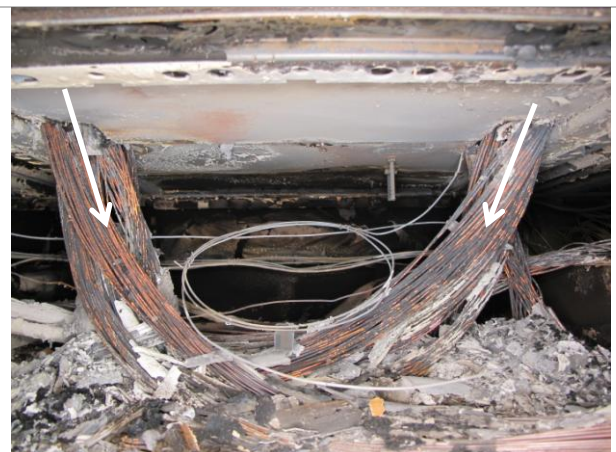
Fig. 37: Central part of the false floor. Arrows showing cable conductors coming from the fire cabinet through the cable passages.
