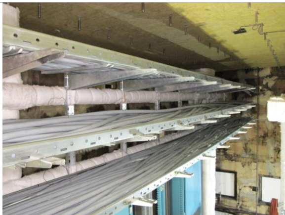
Fig. 4: Overhead cable trays used for CFS-5 to CFS-7 and CORE-6 tests.
