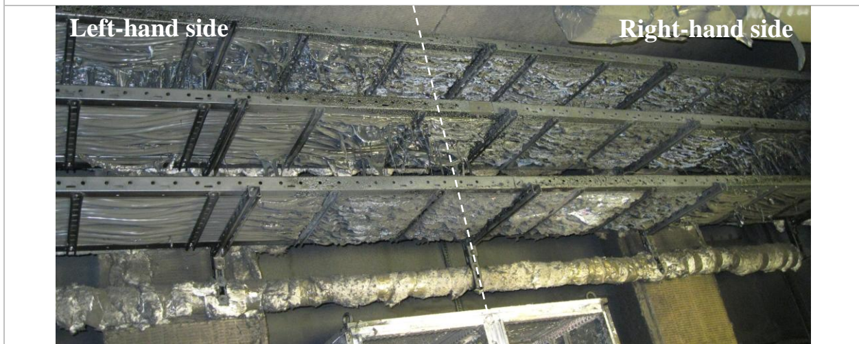
Fig. 24: Global view of the three overhead cable trays after CFS-5 test.
