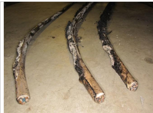
Fig. 36: Samples of cable C (HFR cable-type) contained in the trunking 1 (left-hand adjacent) after CORE-6 test.
