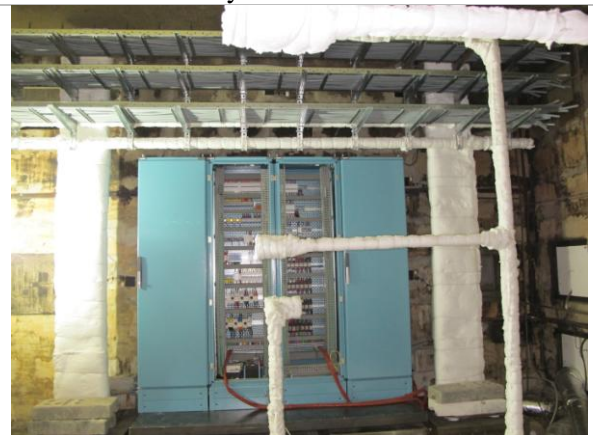
Fig. 5: Open-doors electrical cabinet, adjacent cabinets and overhead cable trays (CORE-6).
