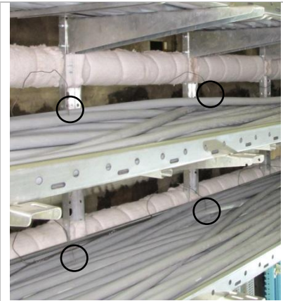
Fig. 11: Thermocouples located just above the cables (circles pointing out their extremity).
