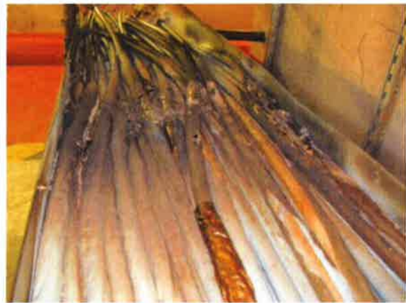
Figure 16: cable samples contained in the protected lower cable tray after the CORE-2 fire.
