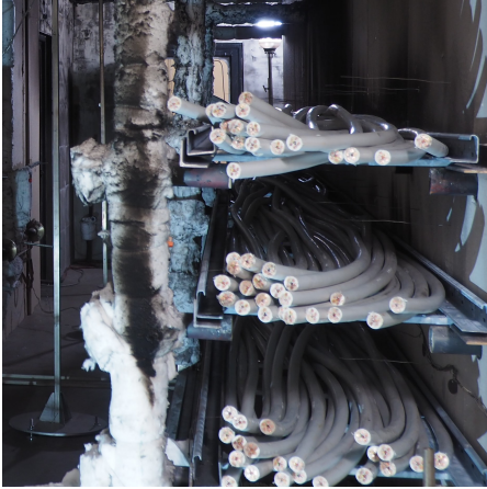
Figure 2: Cable-tray installation in the corridor of the DIVA facility. In this photo, we note the loose arrangement of the 21 PVC cables per tray.
