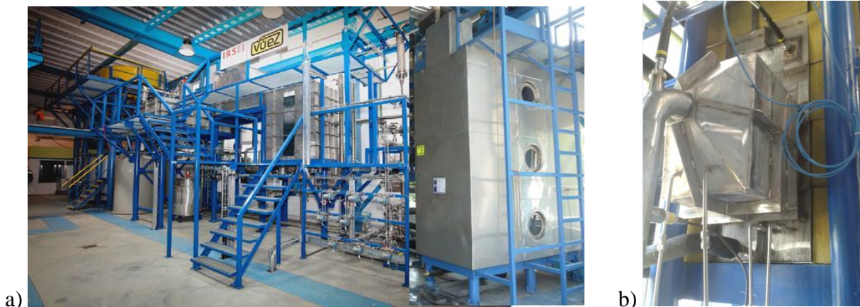
Figure 3. The VIKTORIA facility (a) and the implementation of the strainer (b)
