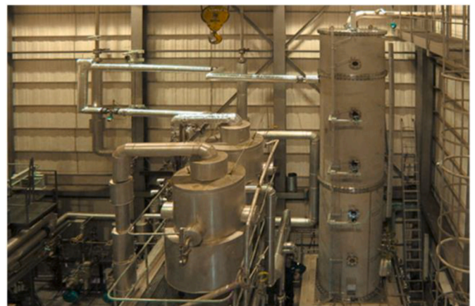
Fig. 4. WP3 - PKL SG No.1, SACO and pool – components and mock-up in principle (primary side not shown).
