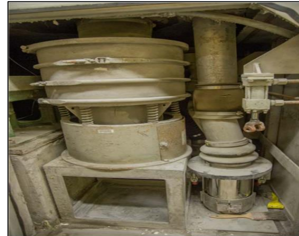
Fig. 1 Sand separator (left) and slag chute with can (right)
